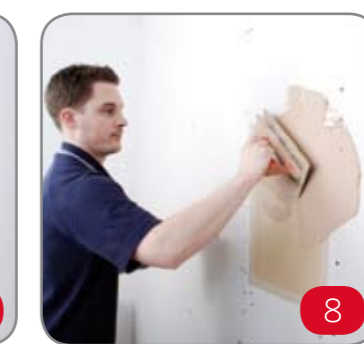
8 Skim with plaster (ordinary multifinish is fine). The best finish is produced when the entire wall is skimmed at the same time. Allow plaster to dry thoroughly before using and before decorating with paint or wallpaper.
